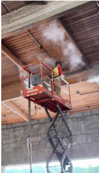
Concourse/ Platform- Ceiling Dry Ice
