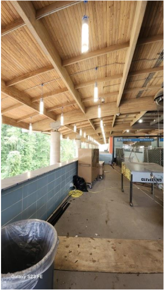
Concourse- New Lighting
